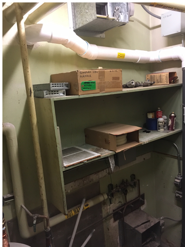
Vent pipe routing in the custodian closet.
