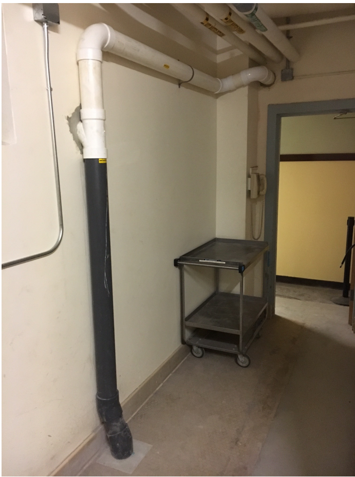
Initial suction in a storage/kiln room adjacent to the fenced courtyard and exterior fan location. Schedule 80 piping was used at the suction points to withstand accidental impacts.
