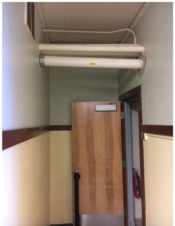
Vent pipe routing from the kiln room to the custodian closet next to the cafeteria and kitchen.
